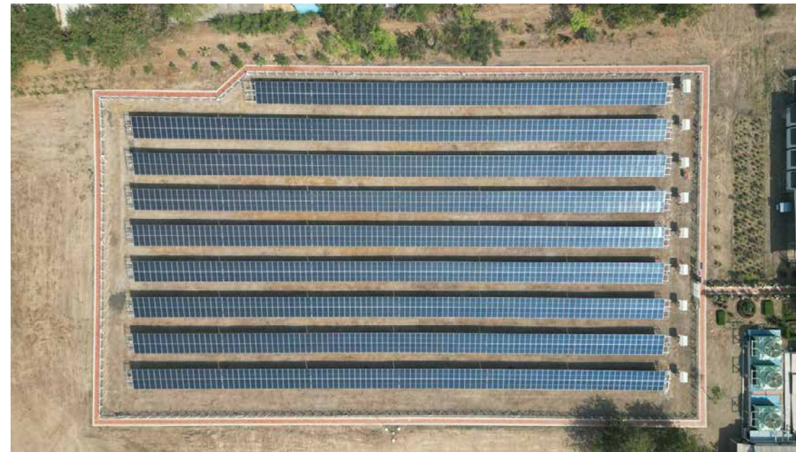
Photovoltaic system at the MAN ES site in Aurangabad (India)
