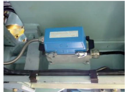
Kistler sensor on engine in operation
