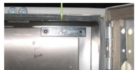
Door stay arm and hinge part has been removed
