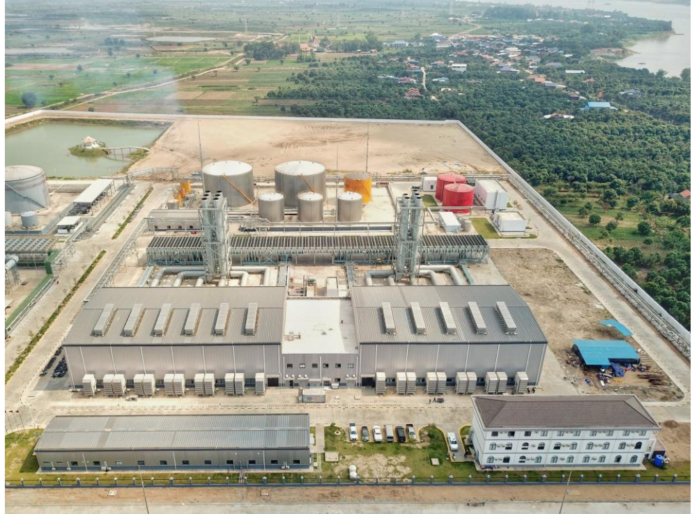
MAN Energy Solutions commissioned a 200 MW power plant near Cambodian capital, Phnom Penh, in April 2021. The plant consists of eleven MAN 18V51/60DF engines (picture courtesy Electricité du Cambodge)
