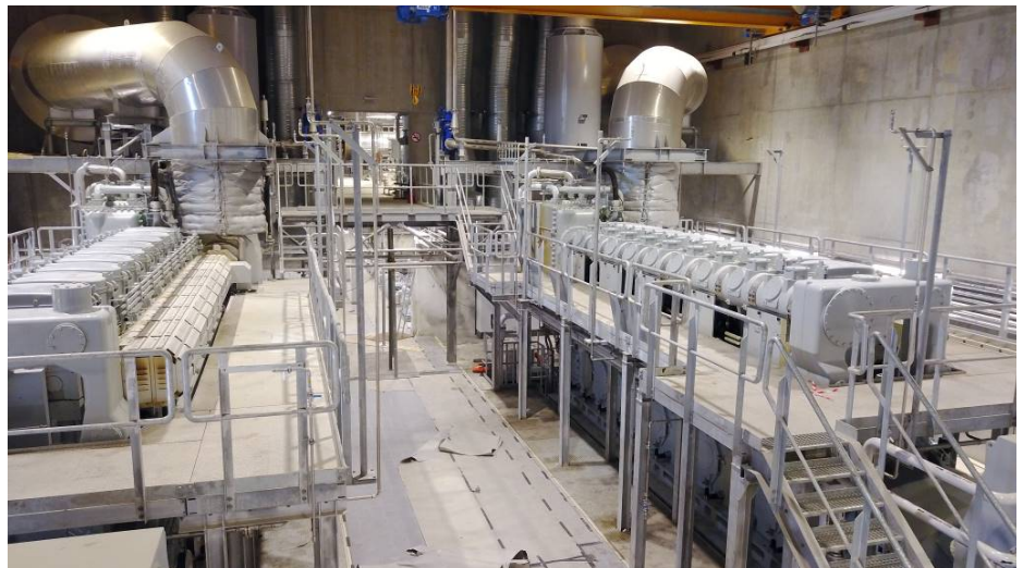
Four MAN 9L51/60 will complement the existing power station with an additional 37 MW power generation, as well as district heating.
