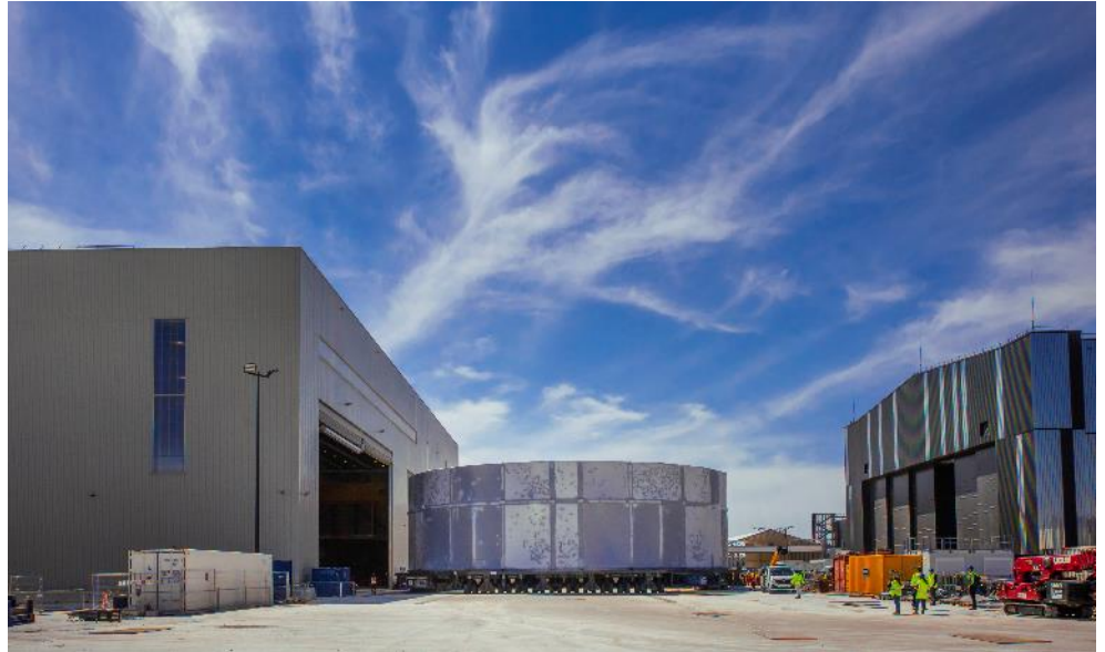
The ,Upper Cylinder‘ leaving the assembly hall at the ITER site in in Cadarache, southern France.
