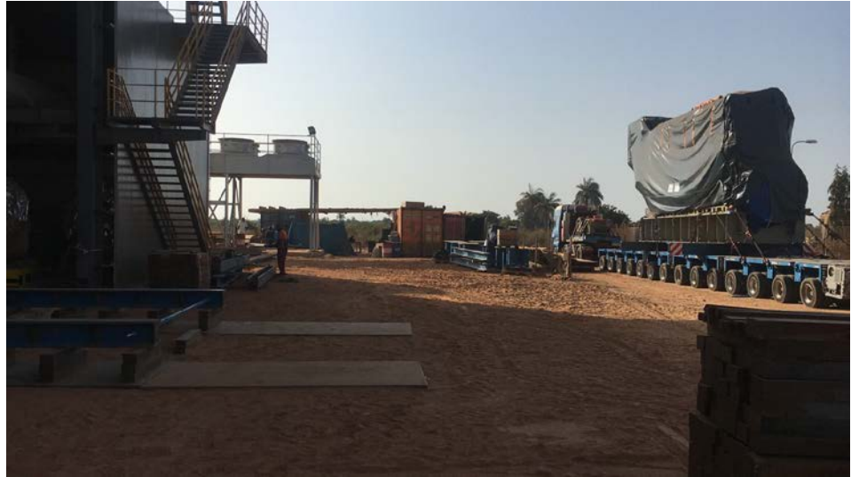
MAN Energy Solutions is supplying two MAN 9L51/60 engines for a newly built power plant in Brikama, Gambia
