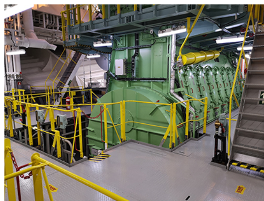
View of the first-generation MAN B&W ME-LGIM engine aboard the 'Mari Jone', the dual-fuel, methanol-powered tanker that Waterfront Shipping took delivery of in 2016. As can be seen, the engine room is noticeably spotless (picture courtesy Marininvest)
