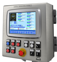
SaCoS control system similar to DF
