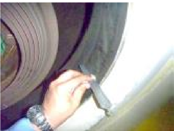
Worn gas outlet guide
