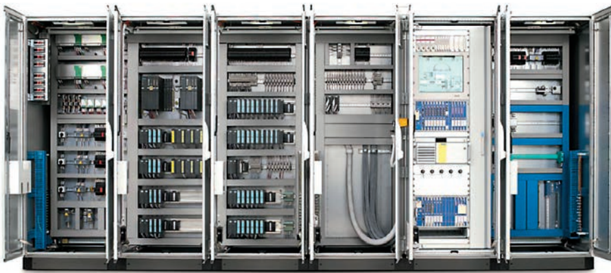
Unit control panel for turbomachinery control
