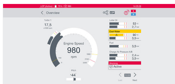
Main overview page of the SaCoS 5000 local operating panel
