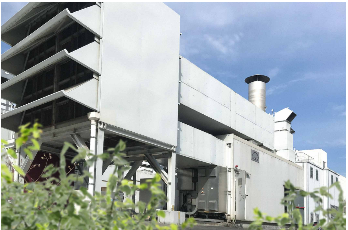
Picture 3 : MGT6000 package installed at SVW site in Shanghai
