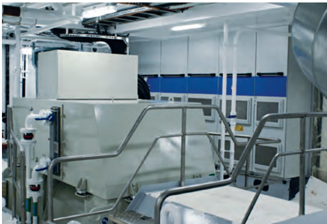
Fig. 14 MAN HyProp ECO in the engine room The shaft machine (PTO/PTI/PTH) is seen in the foreground and the VSD unit in the background
