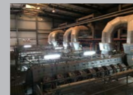
L+V32/40 Existing engines
