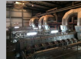
L+V32/40 Existing engines
