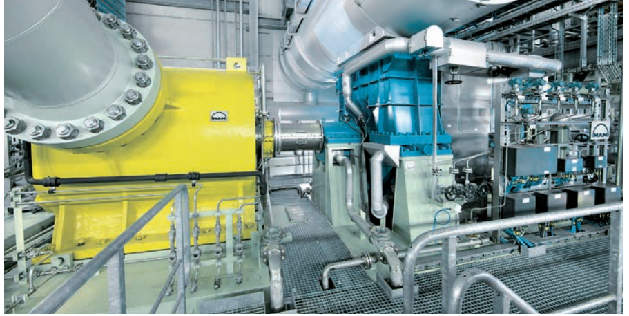
Pipeline compressor and steam turbine. Output: 22 MW
